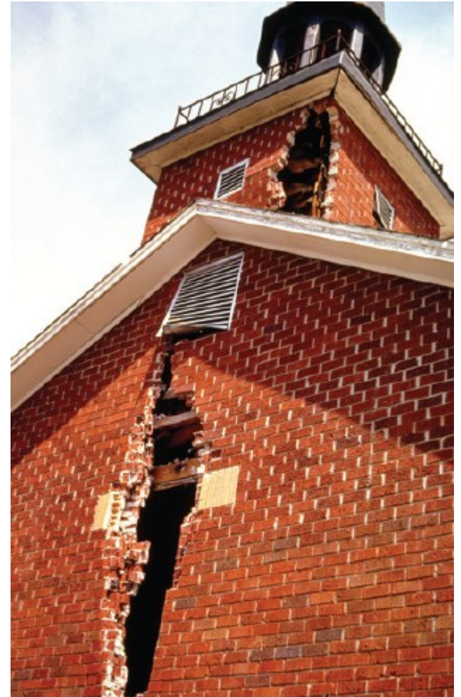
Fig. 4 Damage to a church caused by a bolt of lightning.
